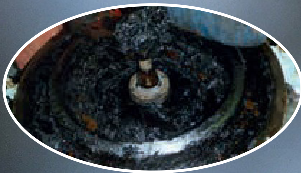
Heavy fuel oil centrifuge overloaded
